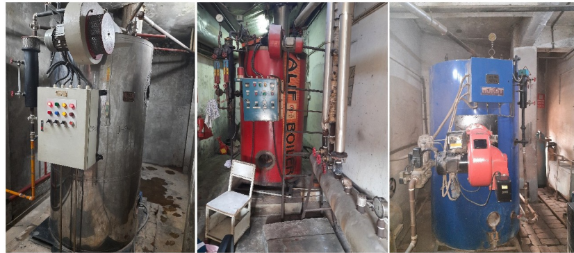
Fig 3. Improper ventilation for the boiler rooms observed during visual inspection.
