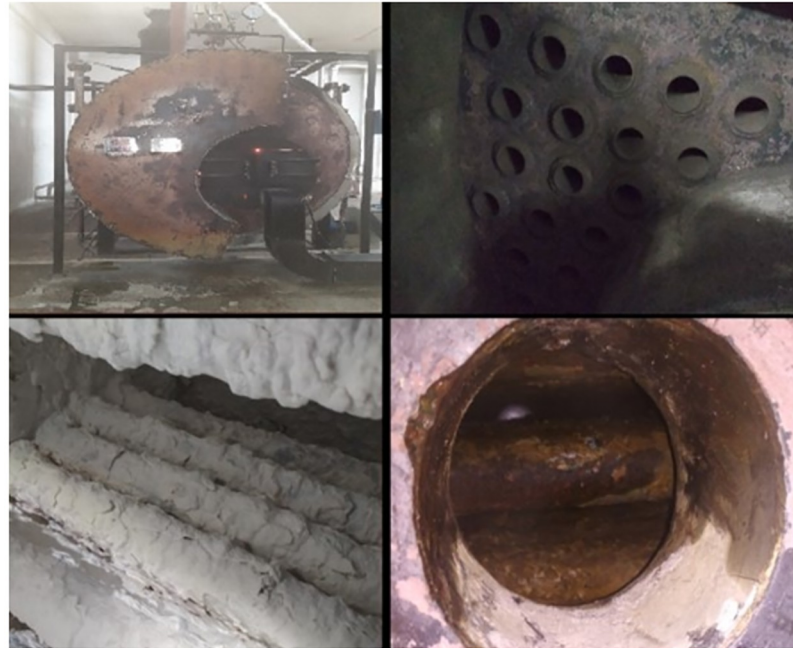
Fig 2. Heat dissipation from an uninsulated heated surface (Top-left), Rusted weld joint and carbon deposit due to unburnt fuel (Top-right), Corrosion of the boiler wall due to calcium build-up from untreated water (Bottom-left and Bottom-right) [39].
