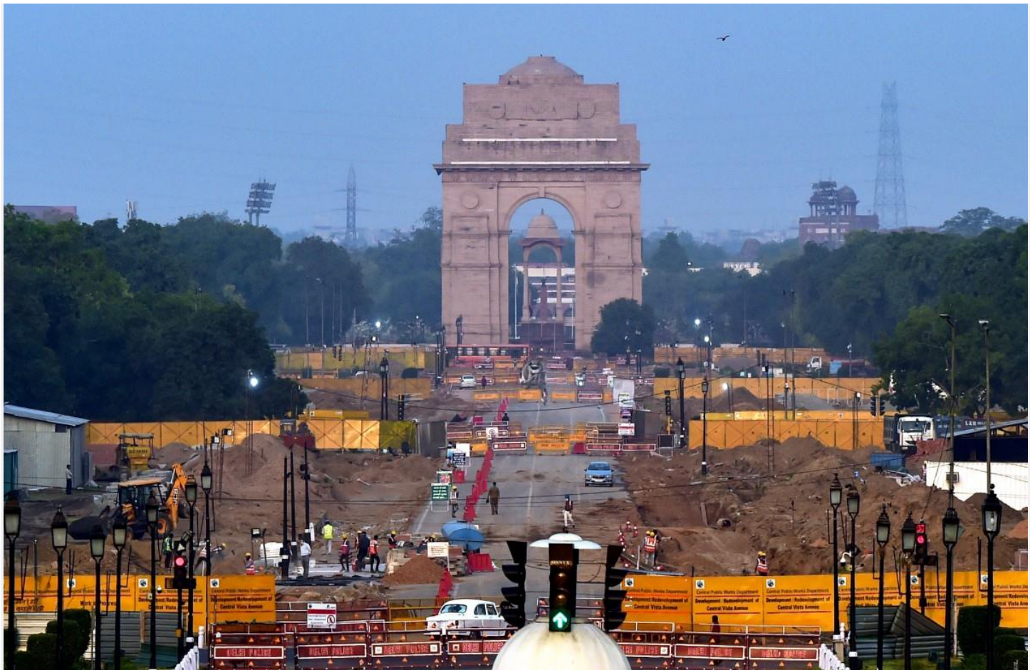
Construction work underway as part of the Central Vista Redevelopment Project, at Rajpath in New Delhi, Friday, May 7, 2021. Photo: PTI/Manvender Vashist
