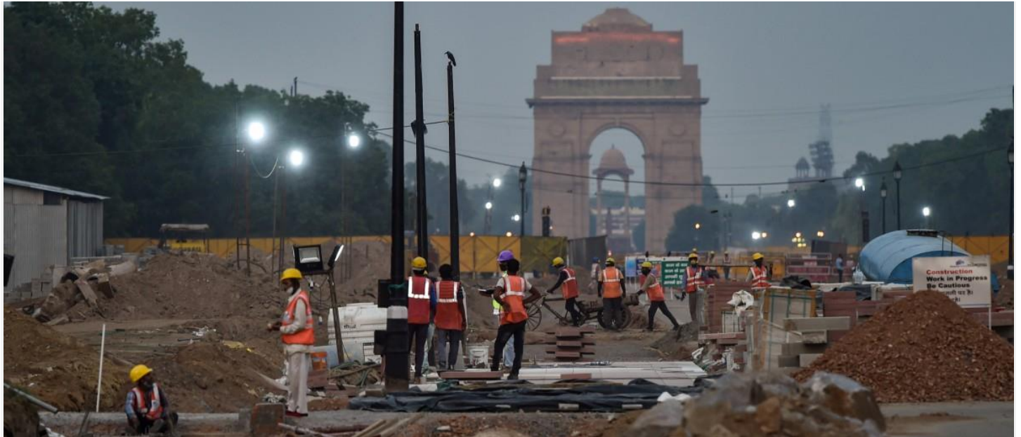
Construction work underway as part of the Central Vista Redevelopment Project, at Rajpath in New Delhi, Friday, May 7, 2021 Photo: PTI/Manvender Vashist
