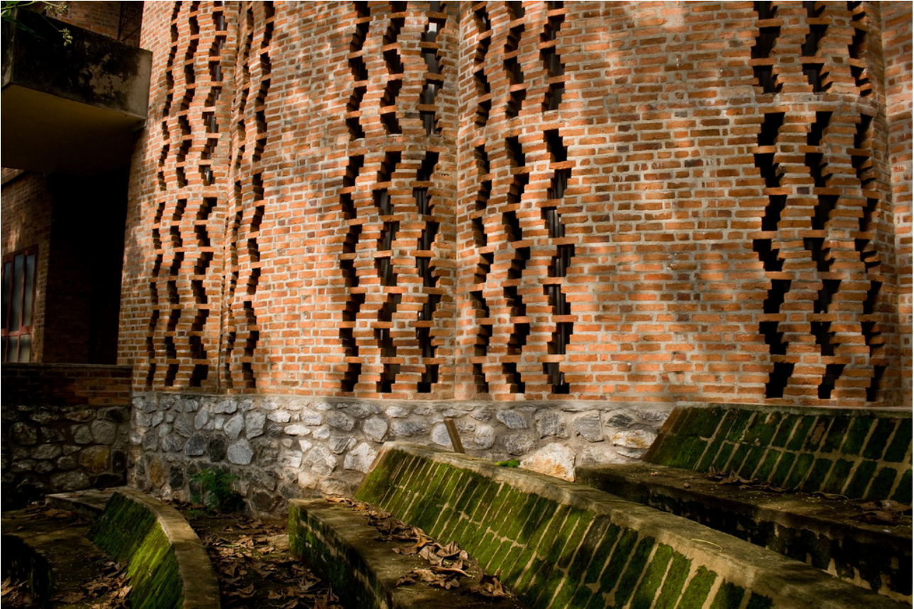
Figure 7: Brick wall at the Centre for Development Studies in Kerala designed by Laurie Baker, (Picture source: http://www.flickr.com/photos/draconianrain/3003397698/ - on a Creative Commons Attribution-Non Commercial 2.0 Generic License accessed August 2013).
