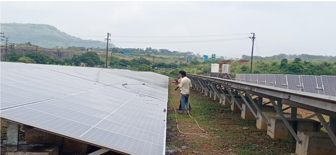
Washing of solar panels. Photo: Divyansh Upadhyay
